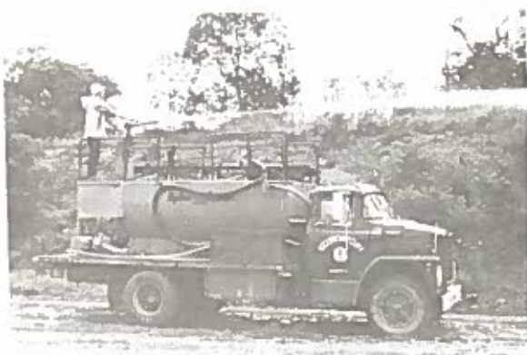
Penn Line Service demonstrates the use of a hydro-seeding unit which combines seed, fertilizer, and mulch in slurry form to achieve rapid revegetation of disturbed areas.
